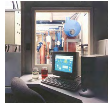
Plant Control Room
