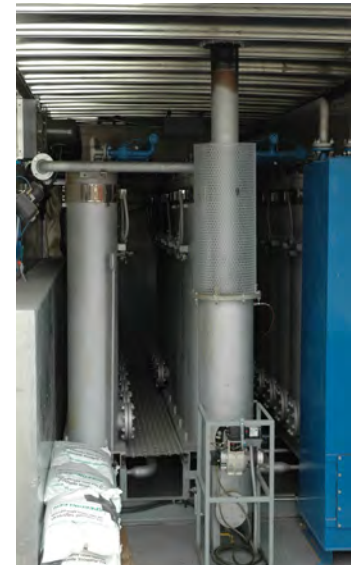
Plant Filtration Columns
