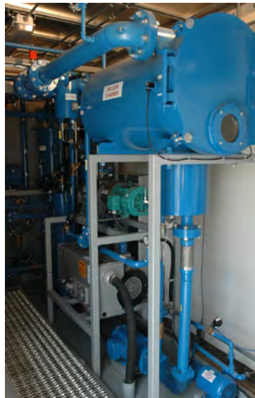
Processing & Vacuum System
