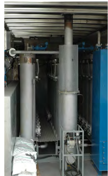
Plant Filtration Columns
