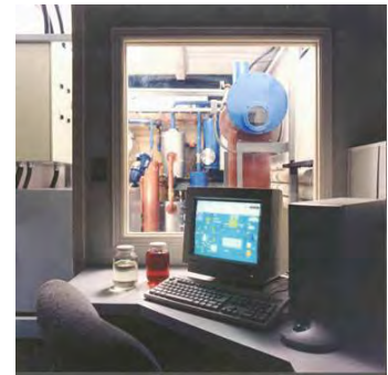
Plant Control Room
