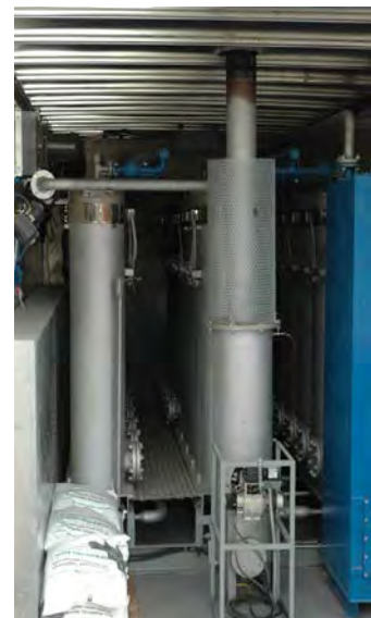
Plant Filtration Columns
